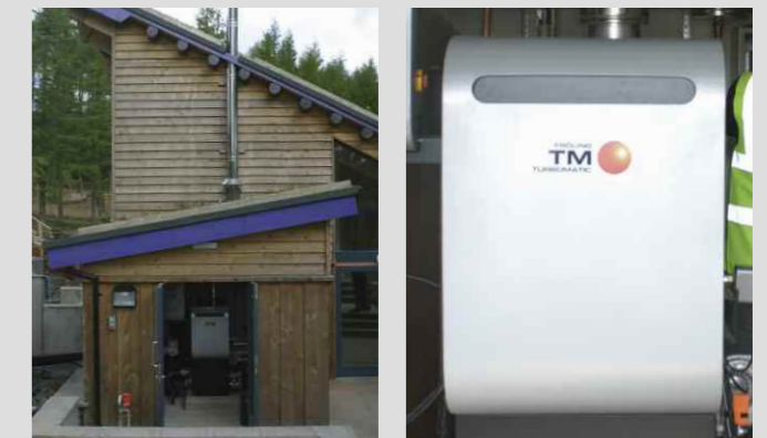
Compact boiler installation integrated with other sustainable technologies
