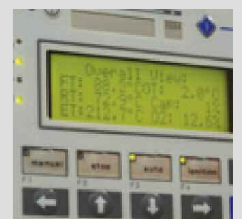
Constant monitoring of water temperature and flue emissions ensures maximum operating efficiency.
